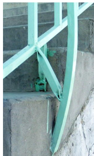
Parwan WRC: Weak support on railing
