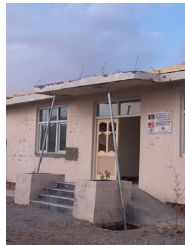
Problematic Construction at Gardez Provincial Women's Center
