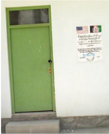
Non-functional toilet facilities with locked door and missing door handle at the Kabul courthouse
