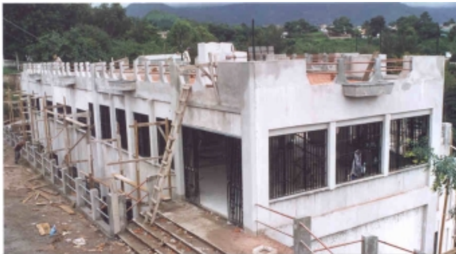
DevTech Systems staff are helping to build and renovate vocational education centers in Honduras
