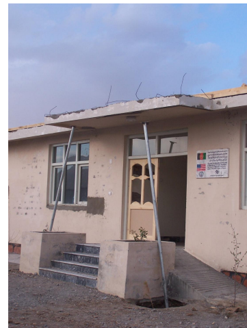
Problematic Construction at Gardez Provincial Women's Center
